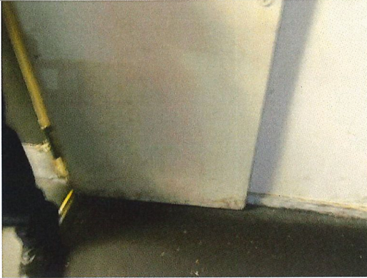
Photo to the left shows the fire door to the kitchen which was nailed open. This practice compromised the escape route
